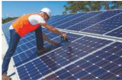
Requirements of the Solar industry
